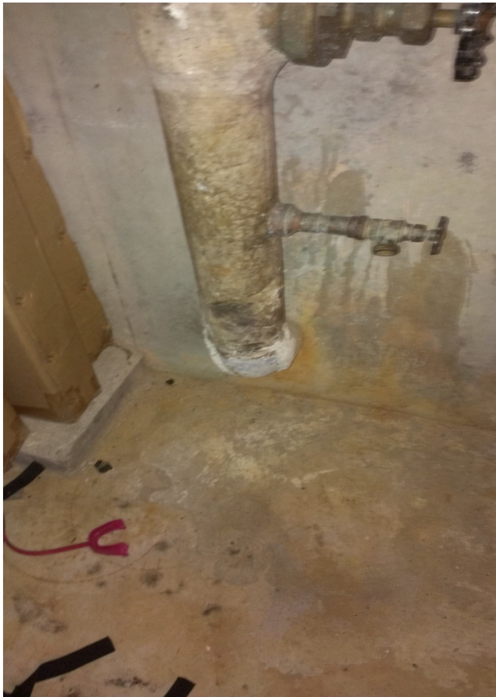
Mudded Elbow and Tee in Mechanical Room
