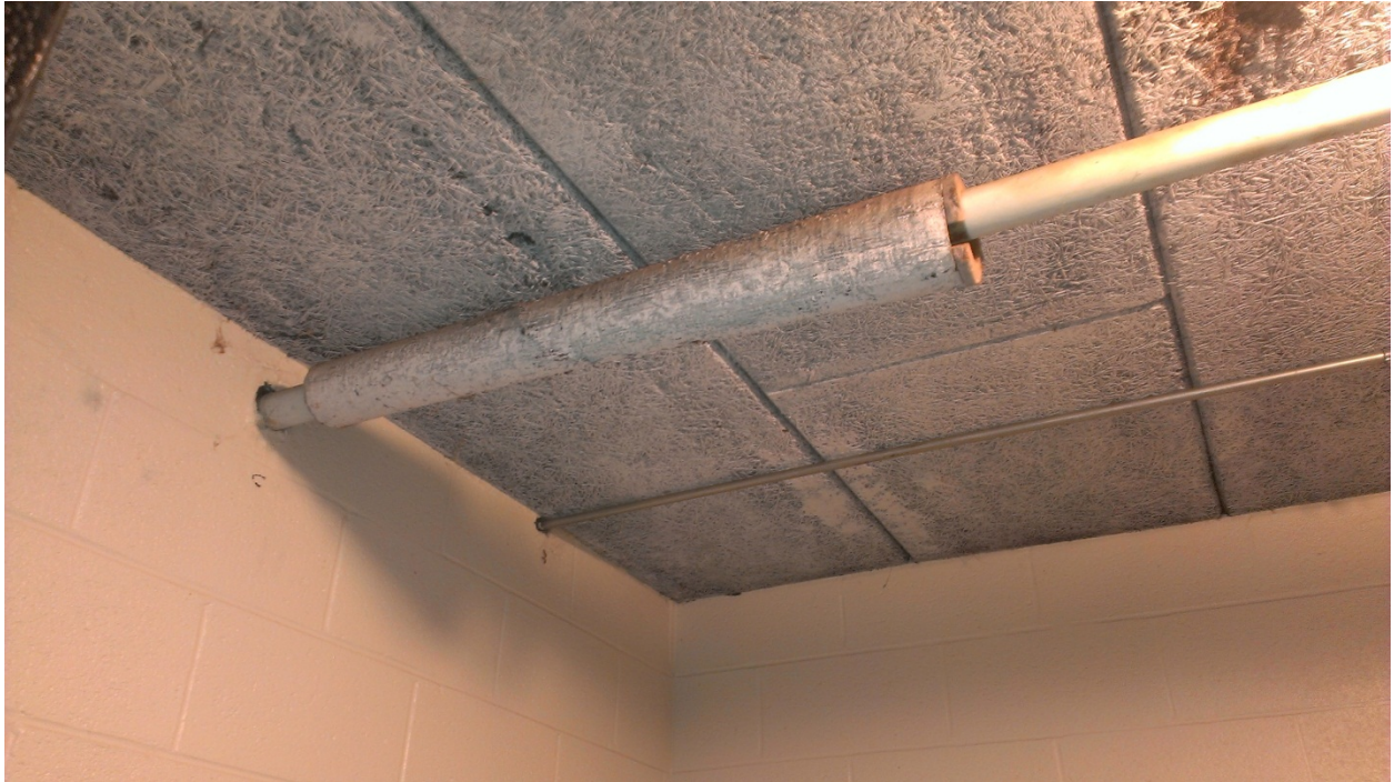
Pipe Insulation in Boys Locker Room
