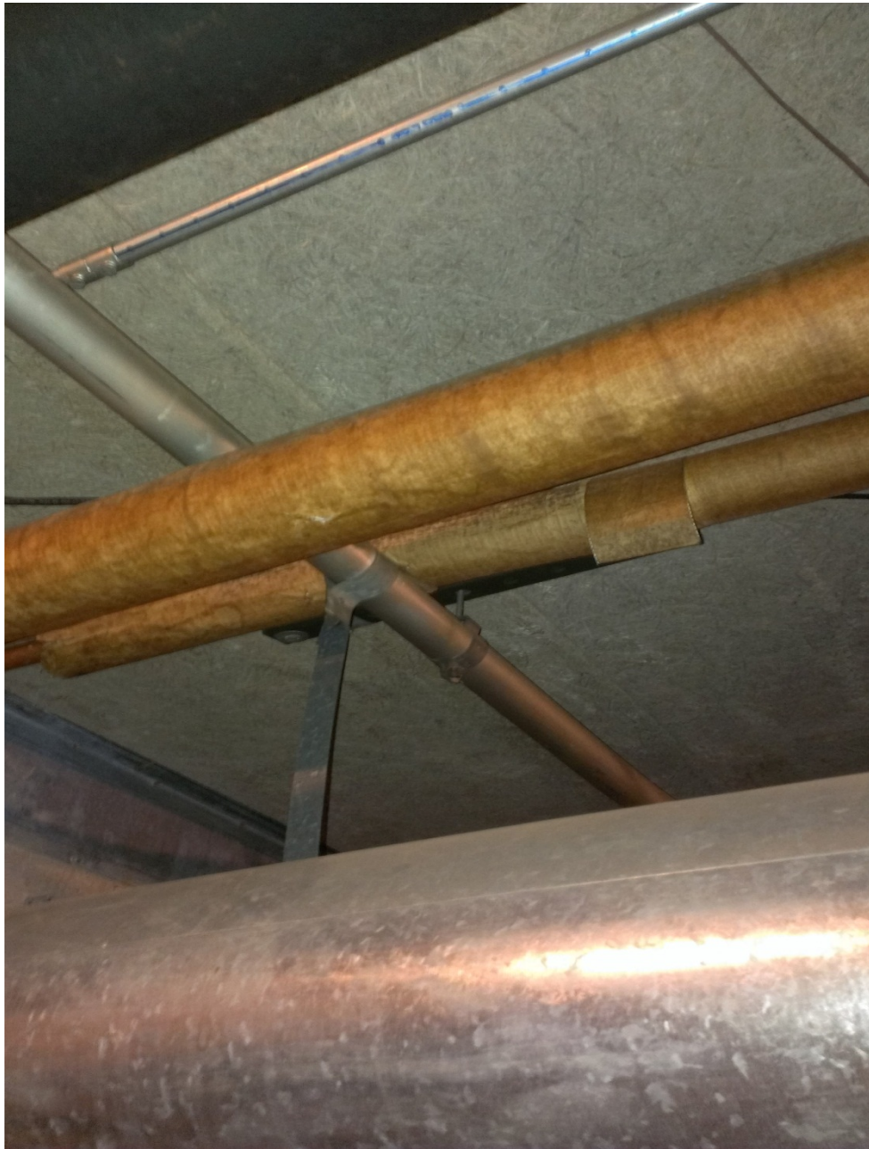
Pipes Run Through the Hall First Floor
