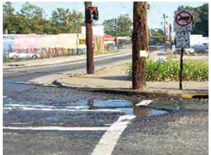
Pavement Conditions at Dill Avenue and Sylvan Road
