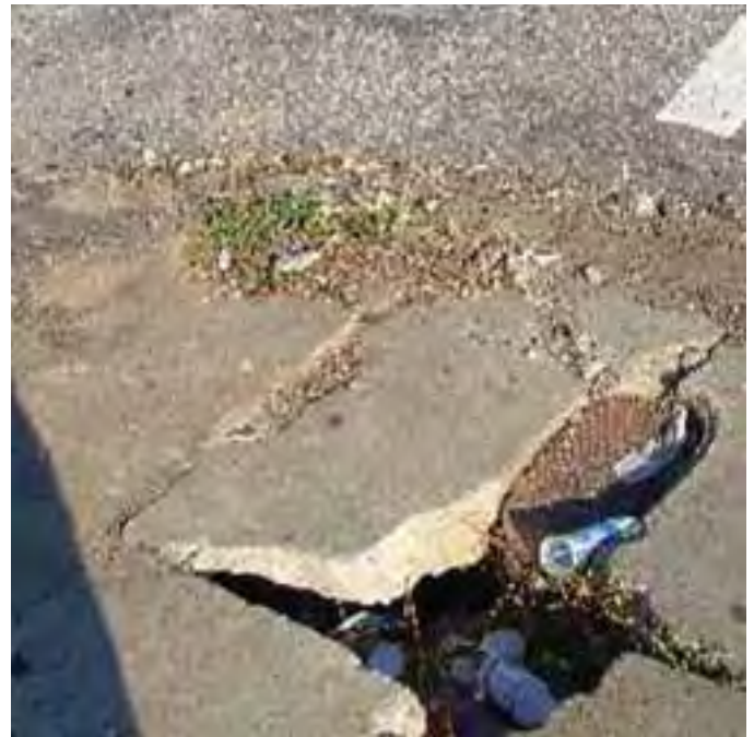
Curb Degradation at Dill Avenue and Sylvan Road
